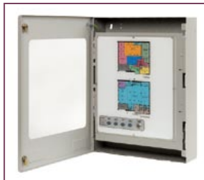
View showing mimic mounted on inner door
